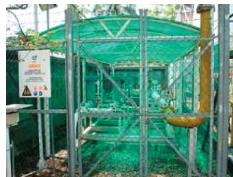
Natural Gas Station
